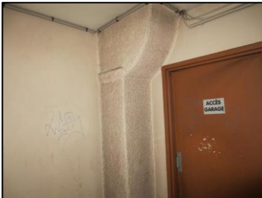
Photo N° 930 AMIANTE CIMENT -- DEGAGEMENT -1 Gainses & coffres verticaux Ventilation haute (Fibres- ciment)
